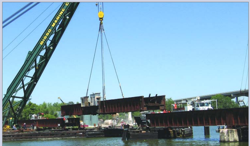
The 200-ton damaged Bayou Boeuf railroad bridge is lifted by an ASA member company and later placed back in place once repairs were completed.
